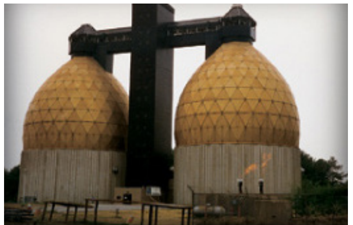
Anaerobic digesters, City of Baltimore
