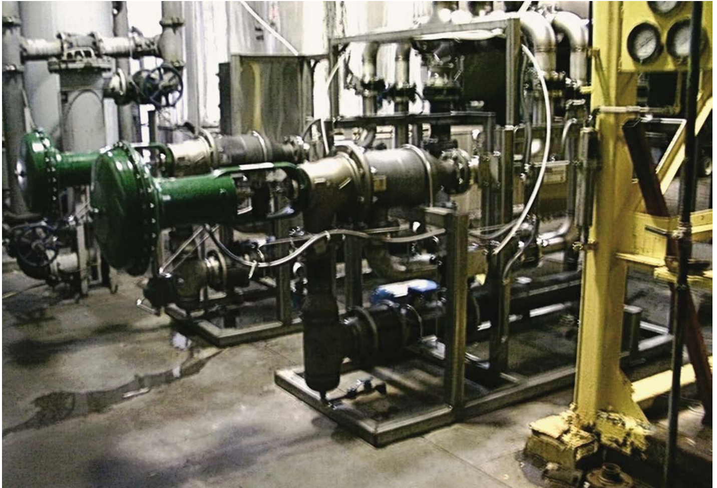
Figure 6: Installed at Creekstone Farms
