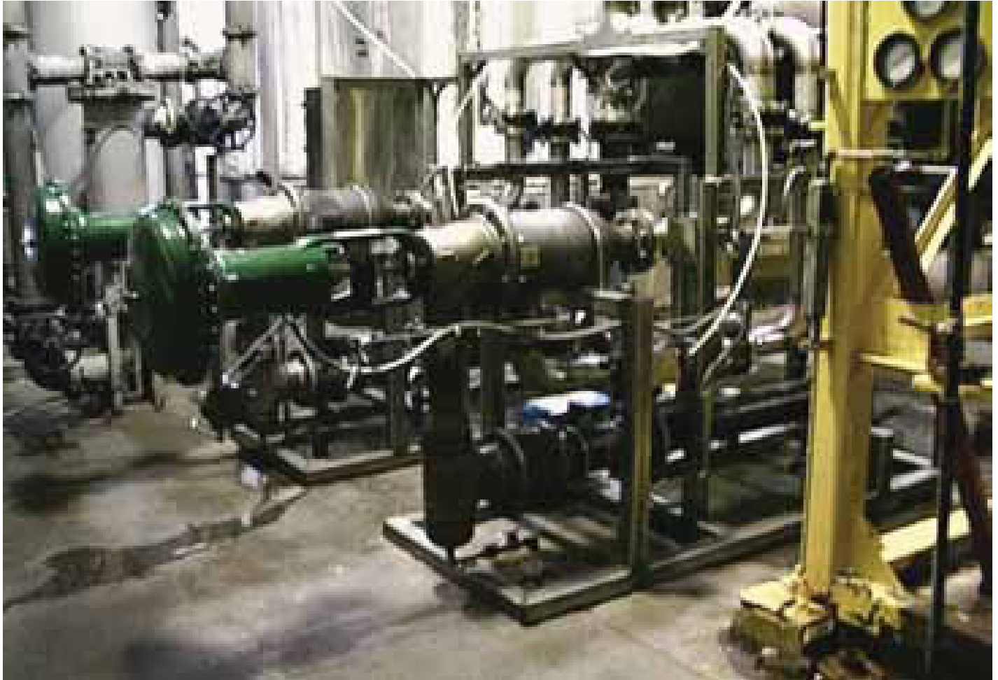
Figure 6: Installed at Creekstone Farms
