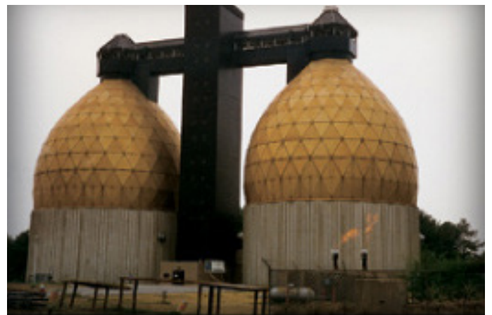
Anaerobic digesters, City of Baltimore
